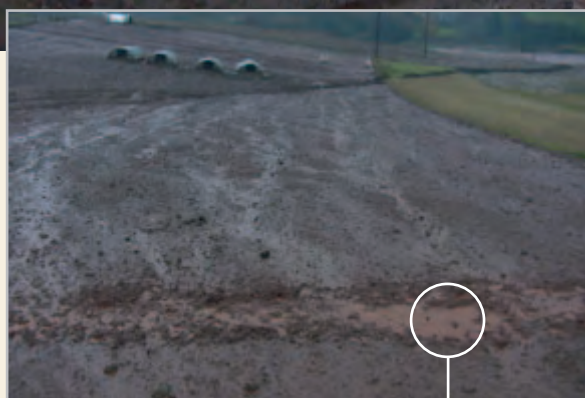
Ponded water and runoff
