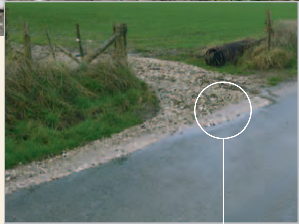
Runoff onto adjacent road
