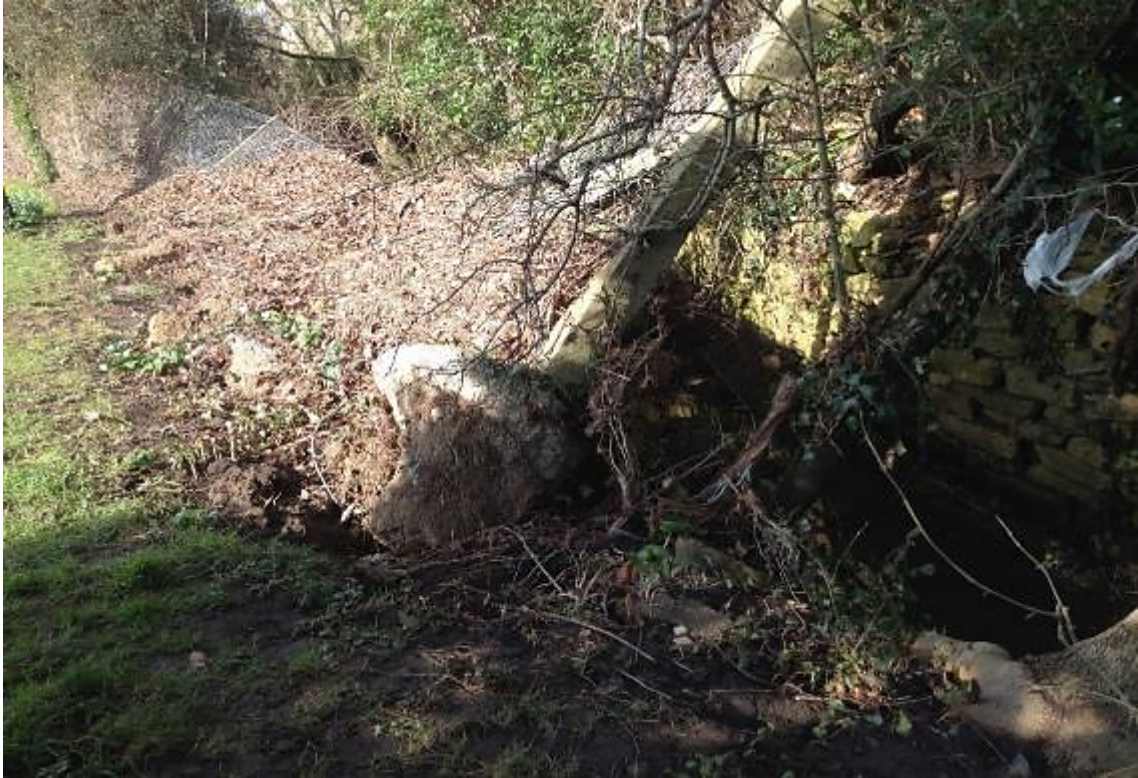
Fig. 5 Martock Recreation Ground - damaged chain link fencing on 06.02.16
