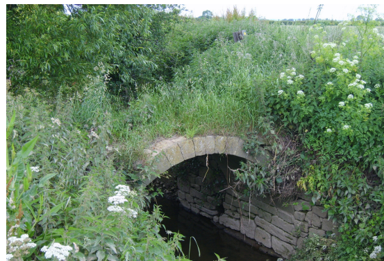
A network of old rhynes drains the low-lying land. Many of the old hamstone arched bridges across them survive. This one takes an old access track over Hinton Meads Brook, west of the village.
